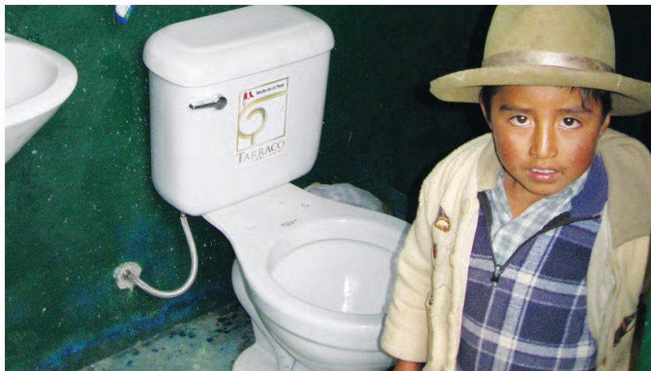
Funding from Deutsche Bank has allowed Agualimpia to help more than a dozen rural communities in Peru to organize potable water and sanitation projects. In the hamlet of Shecta, Agualimpia has installed new toilets and bathrooms for residents.
